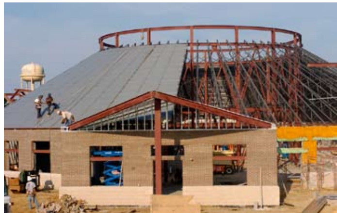
Above: Placement of steel decking to form the roof of the office complex followed quickly after the sloping joists were put in place.
