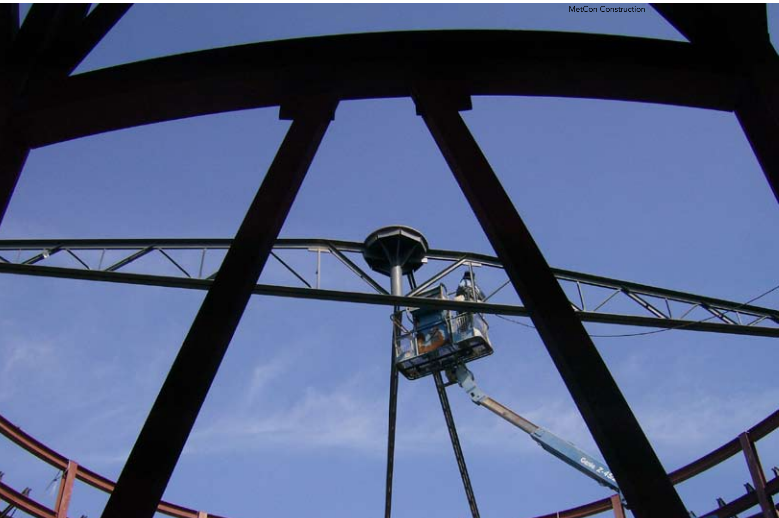
Above: A built-up platform at the center of a 63-ft girder truss provides the upper support for the steel joists supporting the roof.
